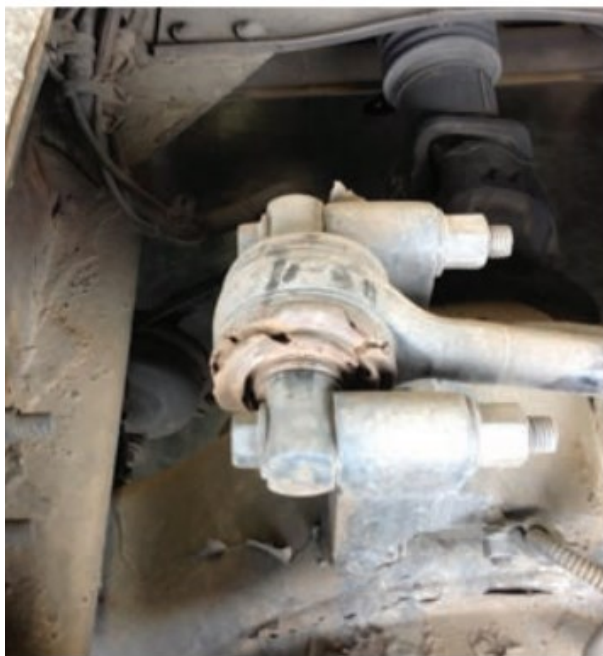
Bushing material is cracked or torn
